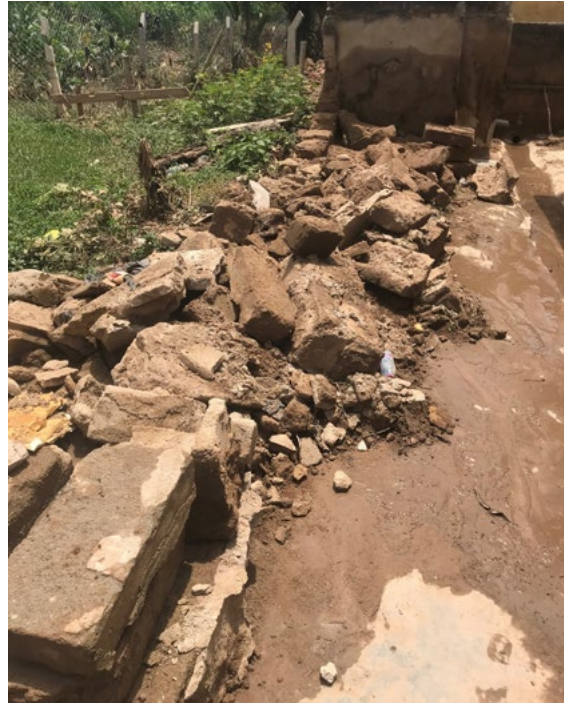
Plate 5: Collapse of a Fence Wall
