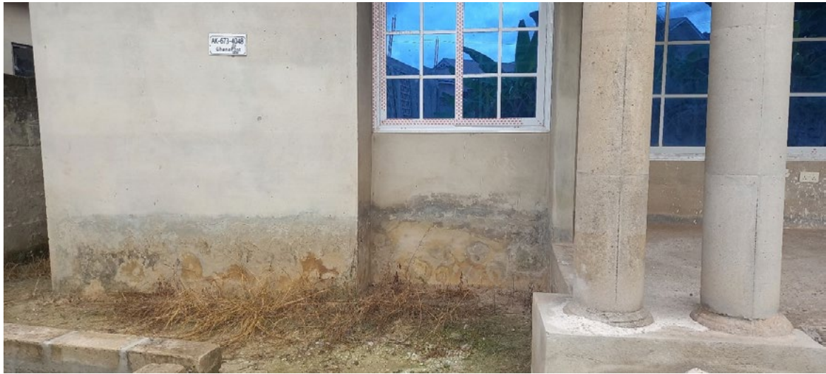
Plate 3 (A): Level of Flood Water Marked on the Walls of Houses
