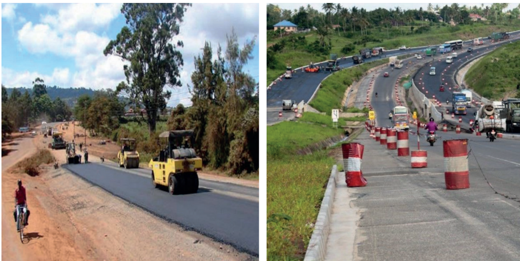
Road construction activities at Luguruni, Dar es Salaam city (Photo by Elitruder during fieldwork in 2020)
